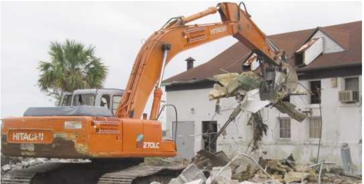
Deconstructing the old base Officers Club helps open the Cooper River shoreline to the rest of the park.
